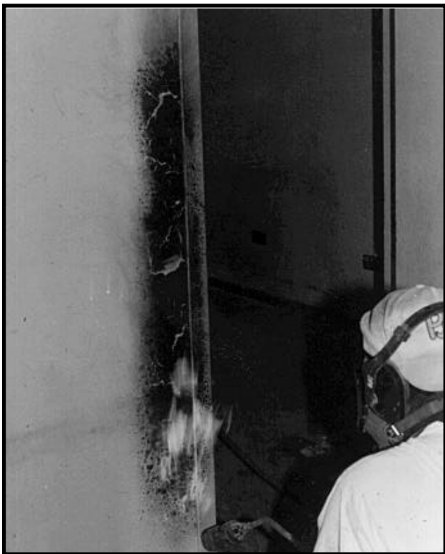
Figure 12.12a Open Flame Burning Is Prohibited.
