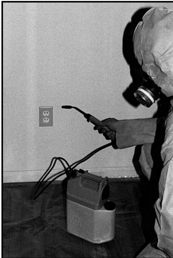
Figure 12.14 Do Not Wet Painted Surfaces Near Electrical Circuits.
