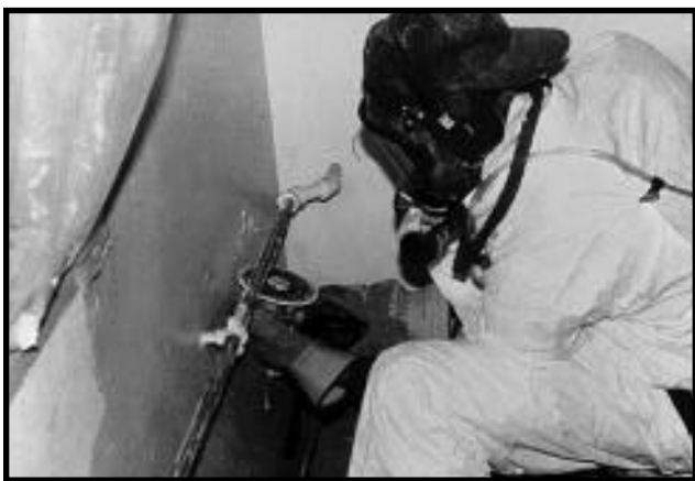
Figure 12.12b Open-Faced Power Sanding or Grinding Is Prohibited.
