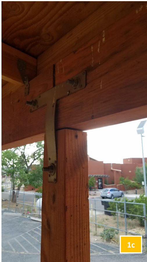
Awning- • (1c) Support beams are separating. • (1d) Support post is separating from beam. • Damaged bracket.
