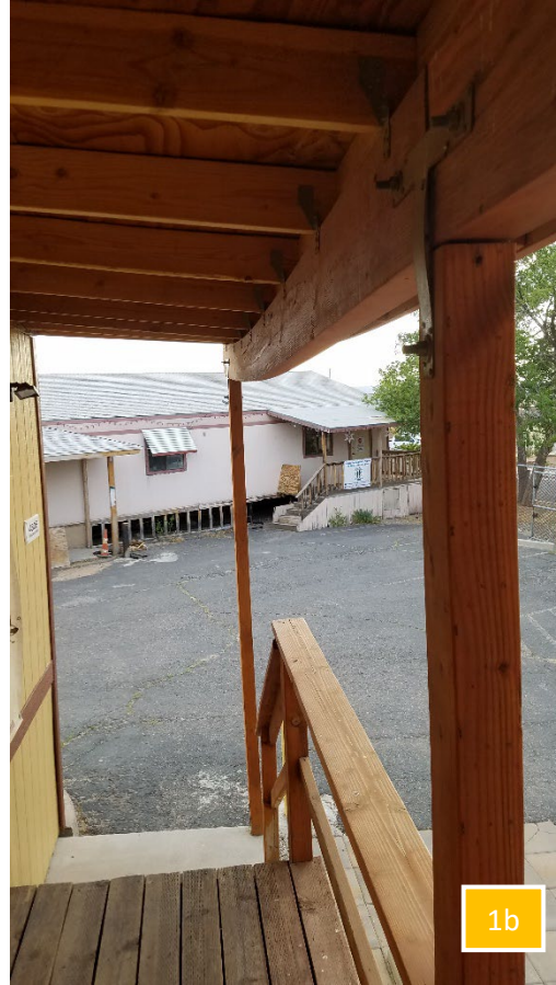
Awning (1a) & (1b)- • Support beam is sagging.
