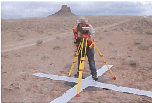
Survey work on the Navajo-Gallup Water Supply Project, a component of the Navajo Nation's water rights settlement in New Mexico. The tribe has a pending water settlement with the state of Utah. Photo: U.S. Bureau of Reclamation
